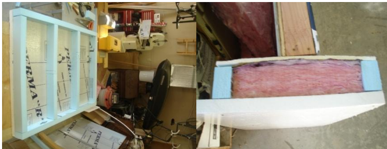
Figure 4 Over-insulated foam walls
